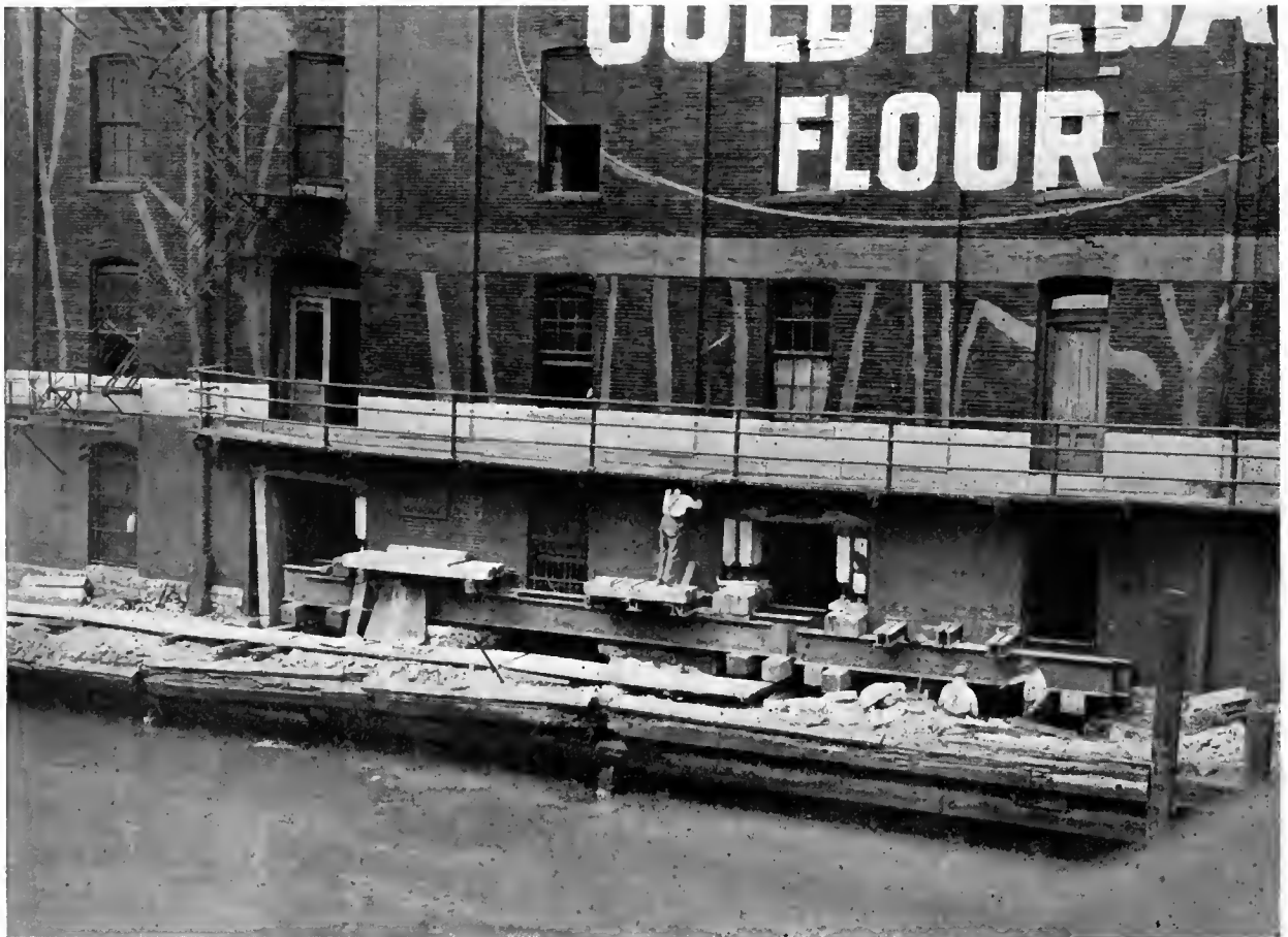
THE CENTRAL WAREHOUSE, CHICAGO Showing the method of raising and supporting the wall during the reconstruction of the foundation
